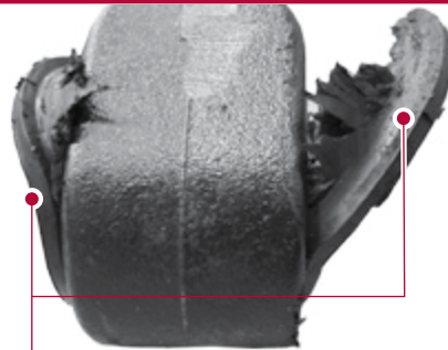
Disconnected Rubber Flange
