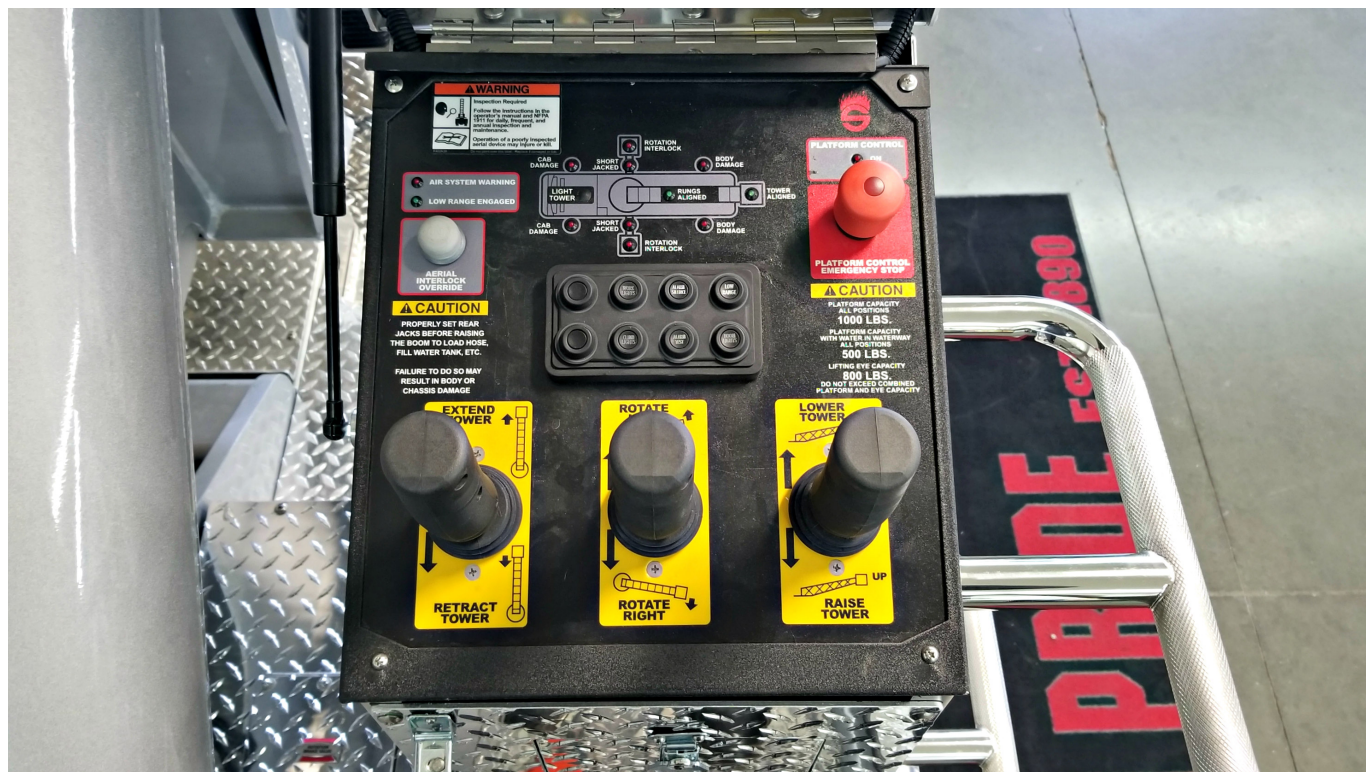
Pedestal Control Panel
