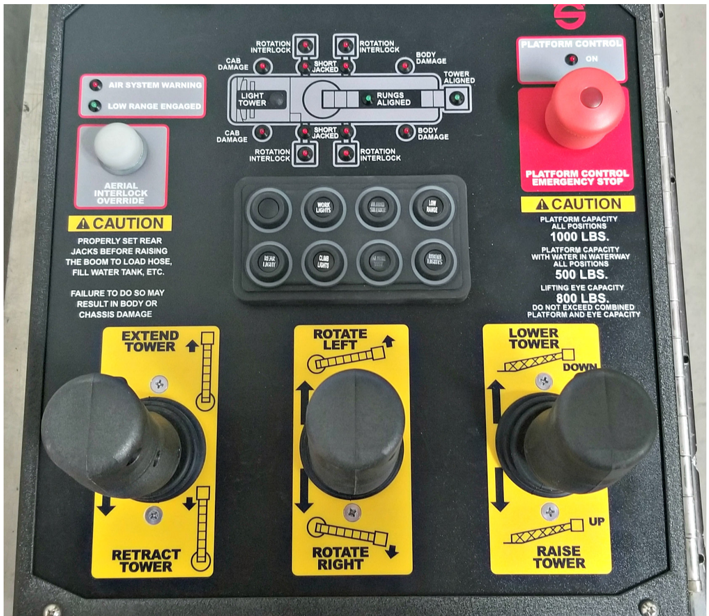
Pedestal Control Panel
