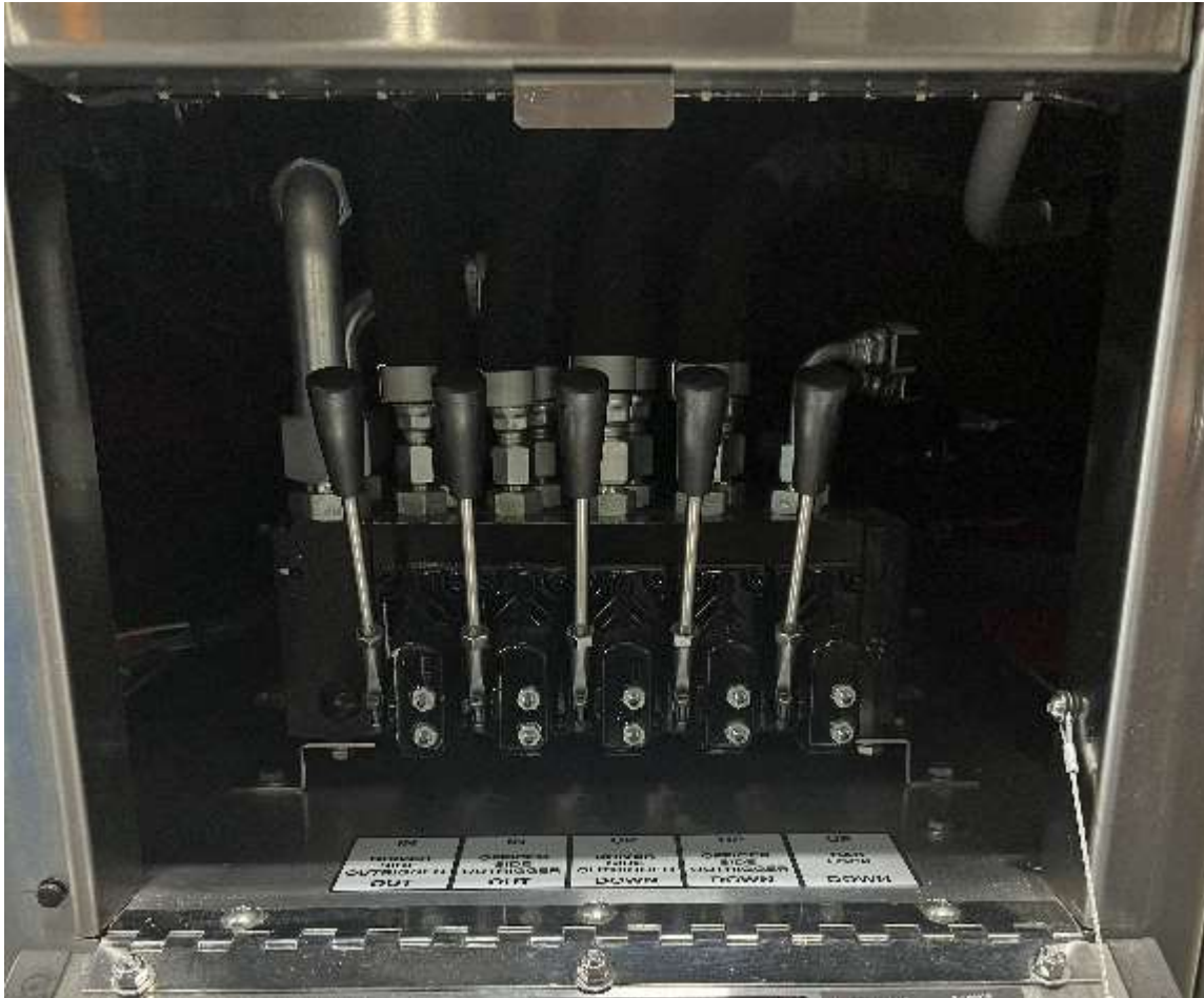
Figure 1- Lower Operator's Station
