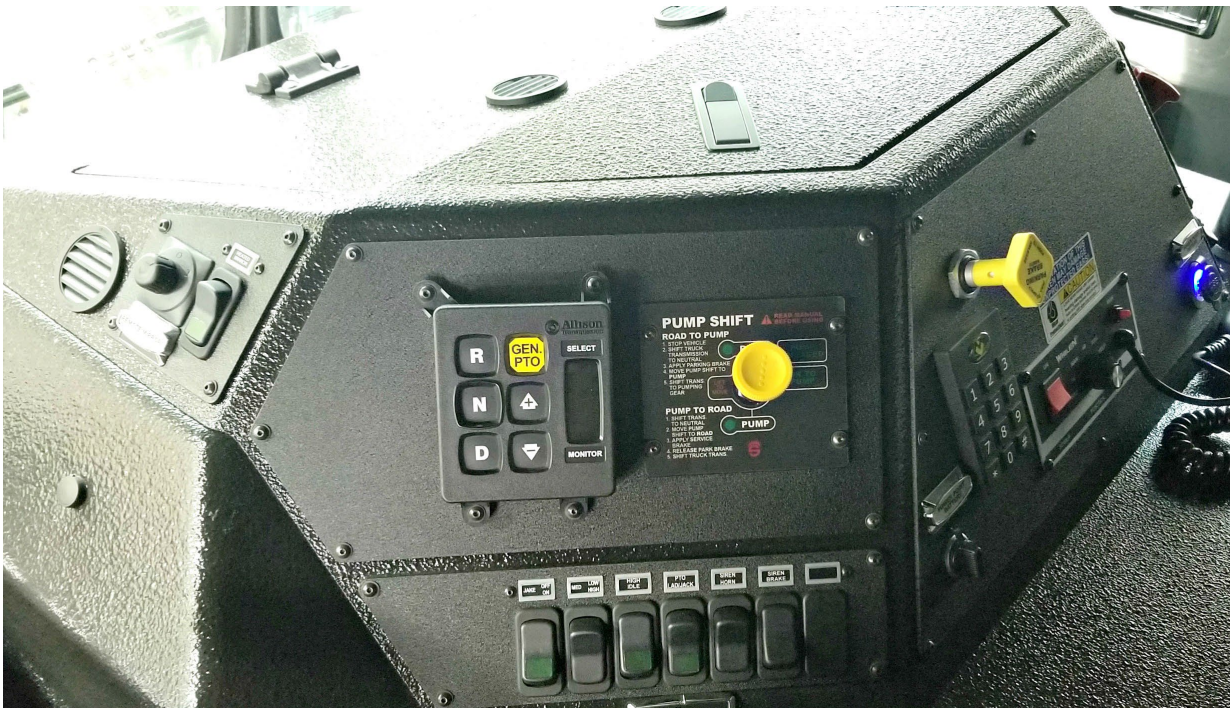
Mode Button and Pilot Light (1) for Generator PTO
